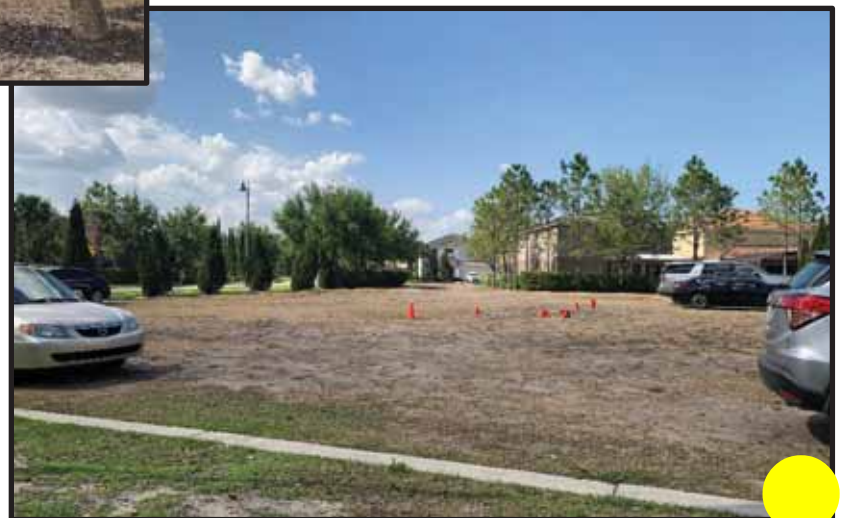
Parking Field is sand trap and needs firm foundation.
